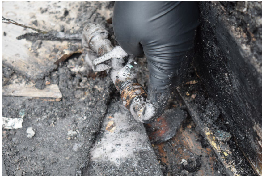
Figure 5 – Soap test on house piping showing bubbles forming near valve. Image provided by MVFD.
